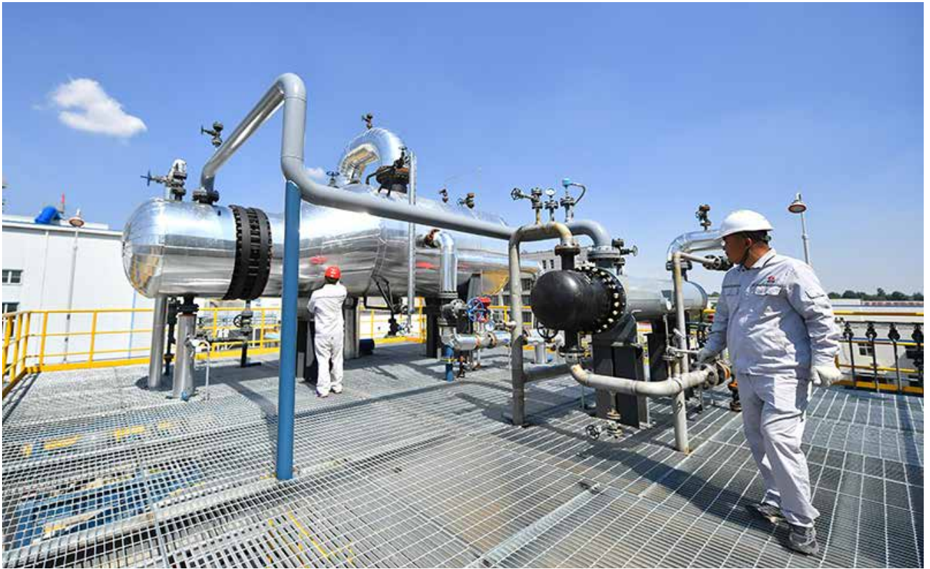
Fig. 2-2 Carbon Capture Facility at Yanchang Petroleum Yulin Coal Chemical Plant, Shaanxi Province (Photo courtesy of Yanchang Petroleum)
