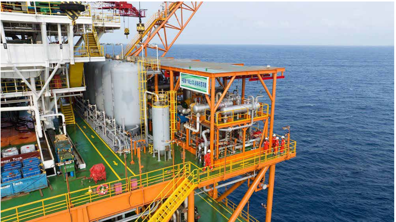
Fig. 2-5 CO 2 processing and reinjection module on the Enping 15-1 Field Platform (Photo courtesy of CNOOC).
