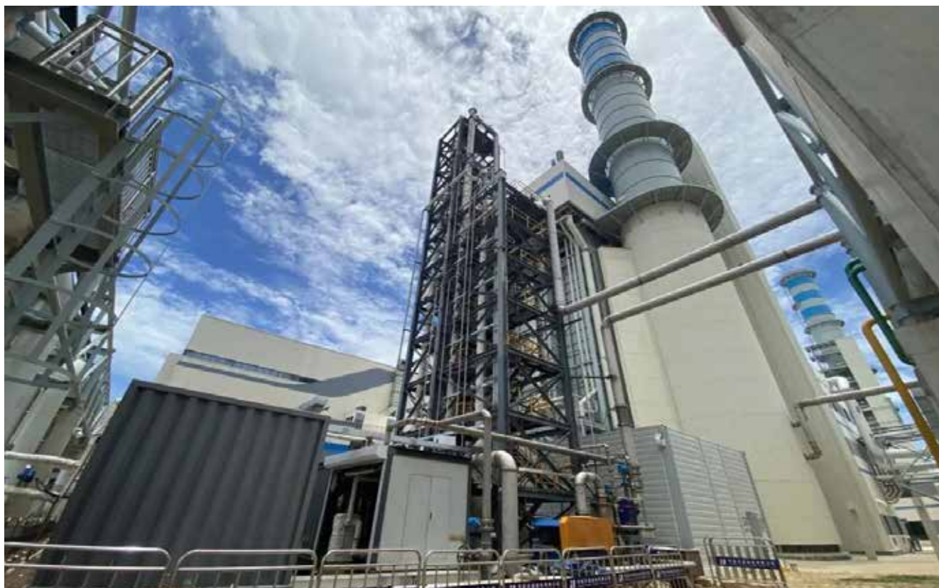
Fig. 2-1 Natural Gas Power Plant Carbon Capture Demonstration Project (2 kt/yr) at Huaneng Yangpu Plant, Hainan Province (Photo courtesy of Huaneng)
